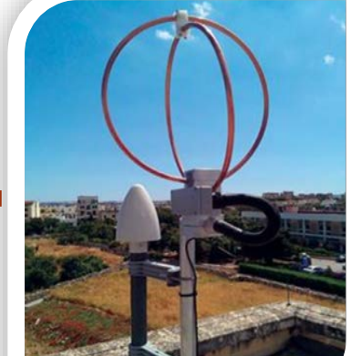
41 Lighting Detection and Tracking System
